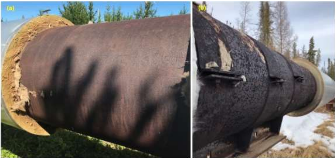
Figure 3-4. Rust scale on the pipe skin for (a) crude oil emulsion pipeline (b) Steam pipeline
