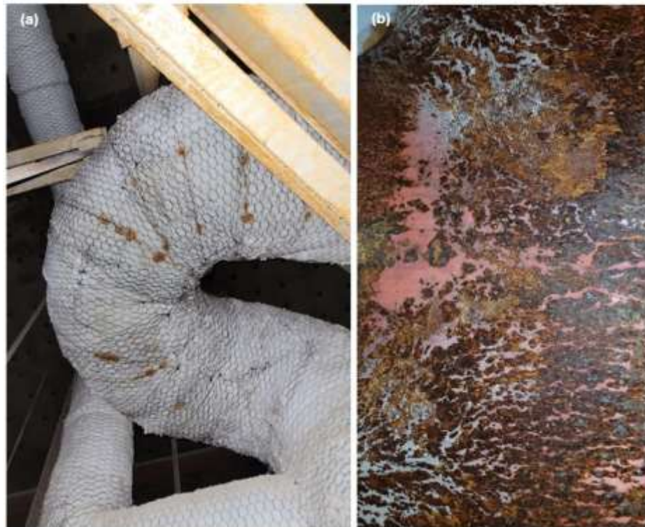
Figure 5-6. (a) Stains on thermal insulation and (b) coating damage & localized corrosion on the pipe skin for the overhead piping
