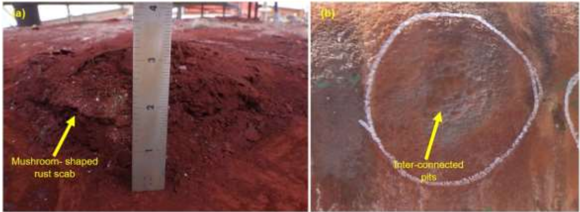
Figure 3-2. Field visuals of the rust scab and underlying inter-connected pits
