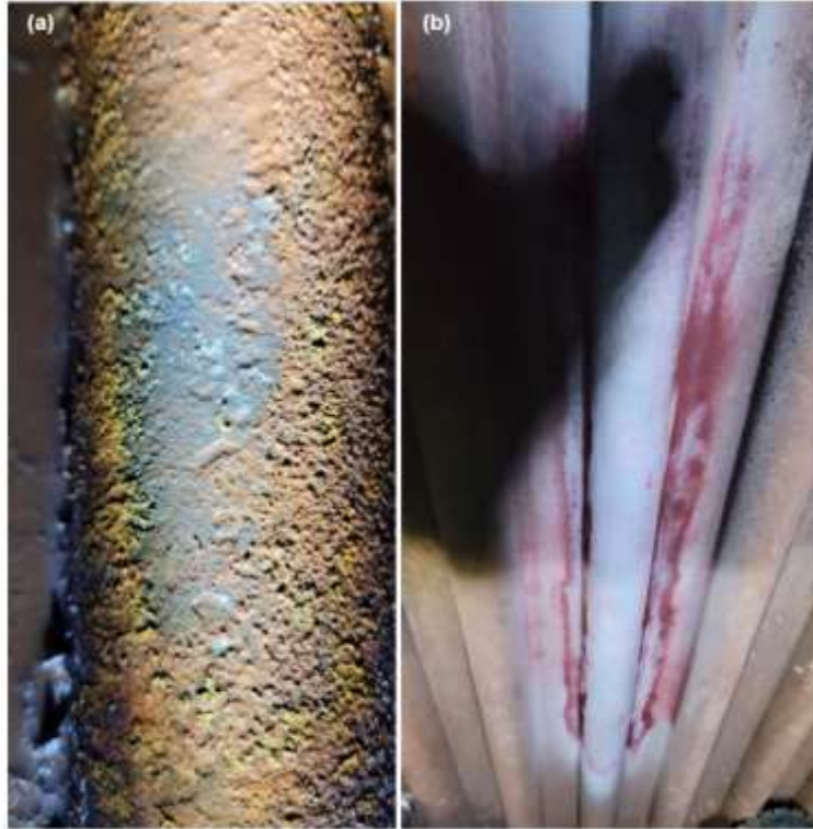
Figure 5-5. (a) Pitting corrosion on the tubes skin (b) Dye penetrant test on the tubes
