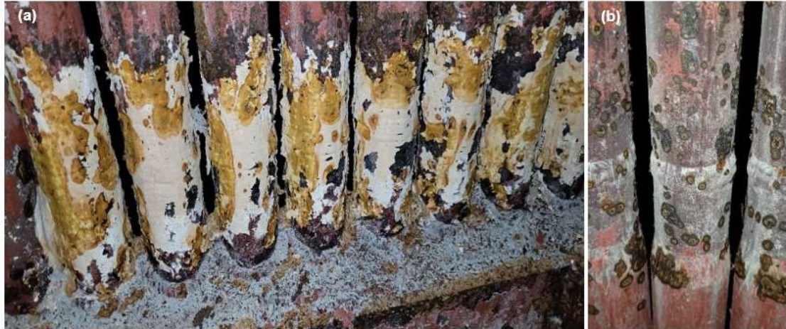
Figure 5-3. Coating detachment and the localized corrosion on the tubes
