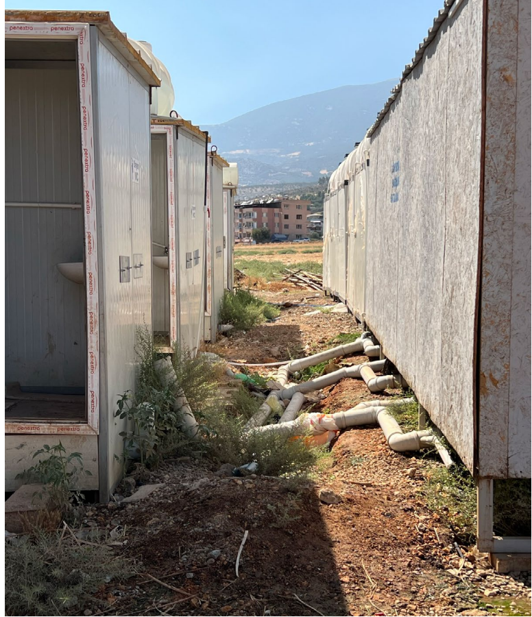
Figure 31. Washroom facilities in camp; septic connections from adjacent buildings are above ground.
