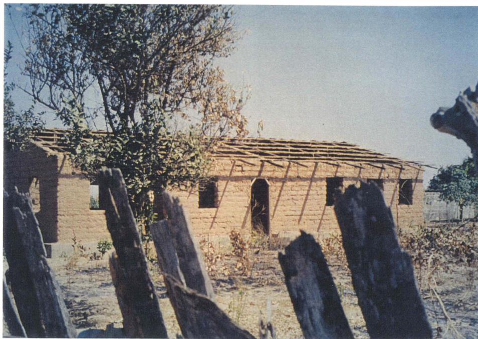
Figure 7a: Compound house construction using local red sand as building material. Split palm trunks form support rafters for metal roof sheeting.
