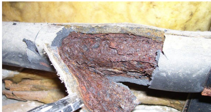
Figure 7 - corrosion under insulation process [14]
