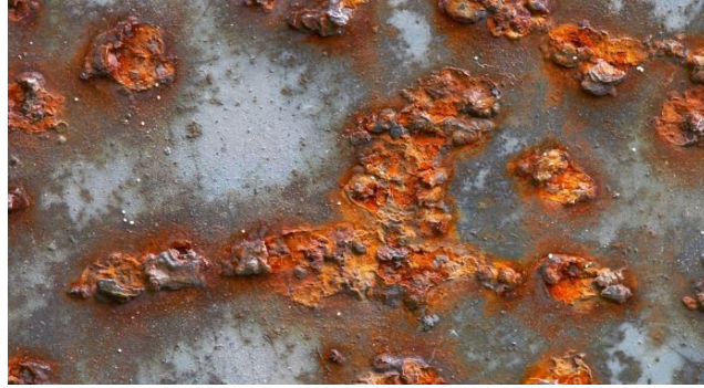
Figure 5 - Localized attack of intergranular corrosion [9]
