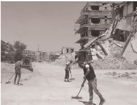
Figure 28. Harasta City Council in cooperation with the civil society carries out asphalt maintenance for a number of Harasta streets (Harasta City Council n.d.).
