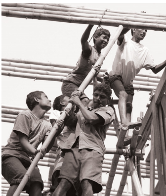
Figure 51. Community members volunteer to build the roof of the METI school (Anna Heringer Studio, n.d.)
