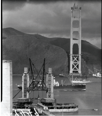
Construction of the Golden Gate Bridge connecting San Francisco to Sausalito, 1935; photographer unknown (OpenSFHistory 1935)
