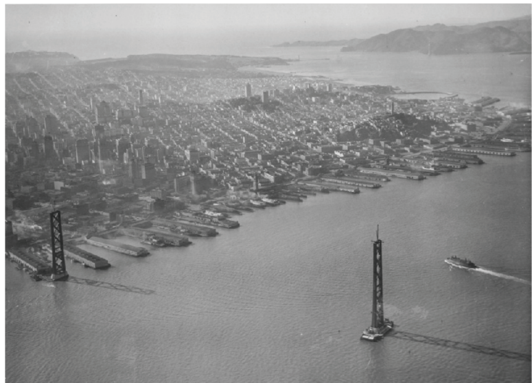
View of Waterfront during construction of the Bay Bridge connecting San Francisco to Oakland, 1934; photographer unknown (OpenSFHistory 1934)
