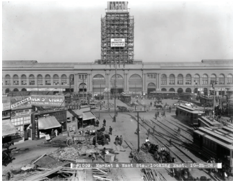
Minor repairs to the Ferry Building while still in use for rescue and relocation efforts, 1906; unknown photographer (Laubscher 2022)
