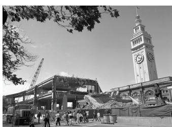
Demolition of the Embarcadero Freeway following the Loma Prieta Earthquake in 1991; photograph by Greg Gaar (OpenSFHistory 1991)
