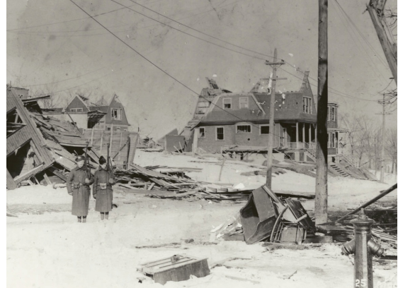
Devastation on Kaye Street near Gottingen Street. The Church site is likely just after the large houses still standing (MacLaughlan 1917 or 1918)
