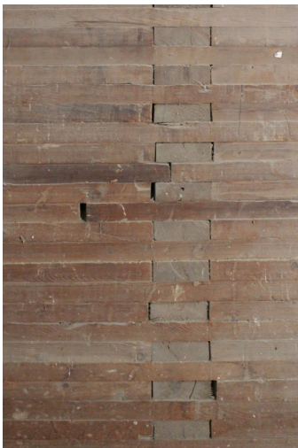
Figure 34: Cribbed construction employs a log cabin technique of laying dimensional lumber flat on top of each other that interlock at corners.
