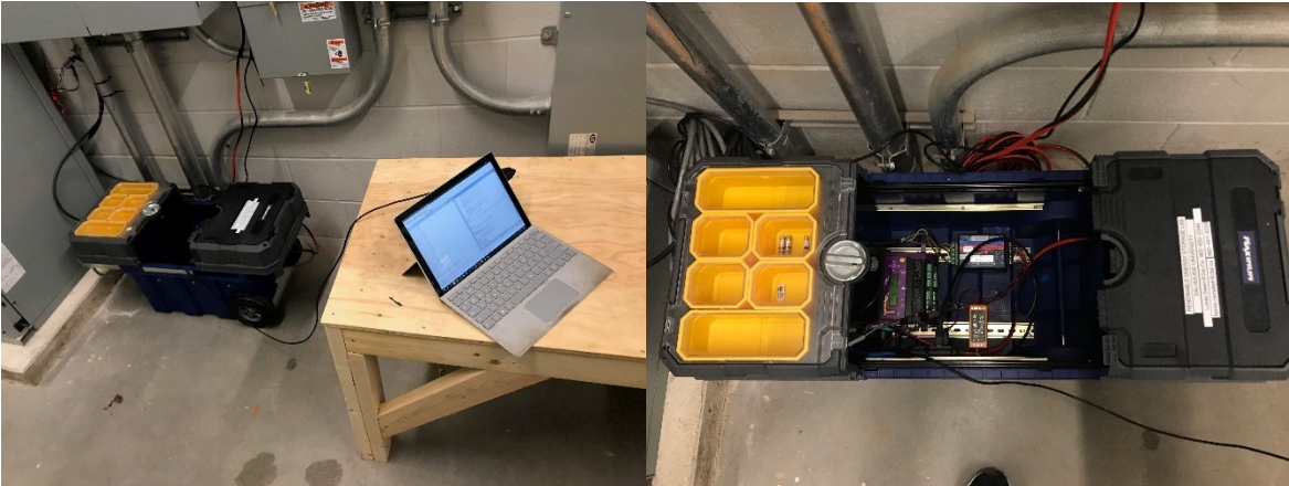
Figure 32. RESL commercial BESS monitoring system
