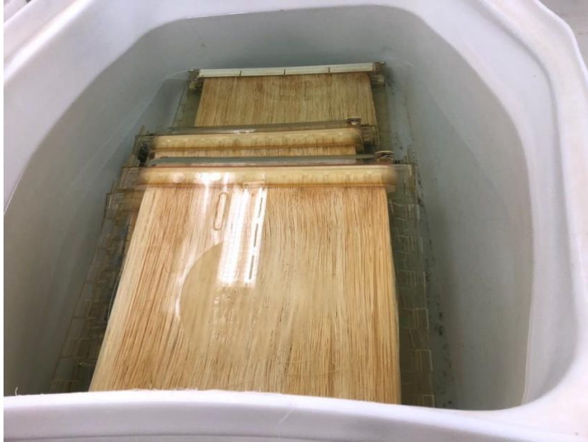
Figure 2 Ultrafiltration membrane cassettes at Pottle Lake Water Treatment Plant. Taken October 2018 by Mikaela Zwicker.
