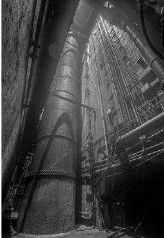
Photo is taken from the Turbine Deck looking up the shaft along one of the penstocks (Conlon 2019).
