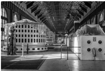
Interior of the Turbine Hall. The eleven dynamos are repeated along its length, with the electricity that they generate being fed into the bus breakers on the right (Conlon 2019).
