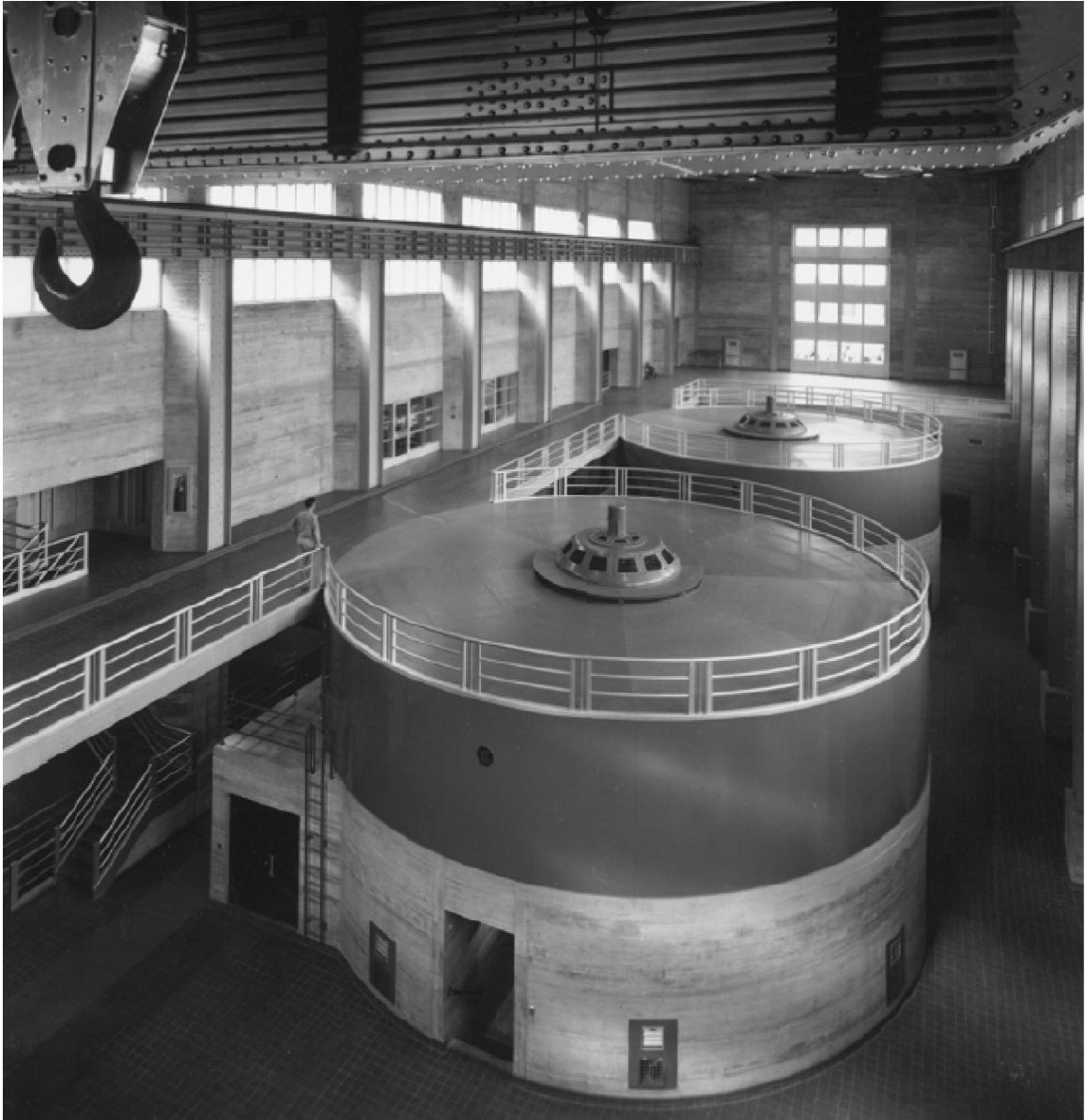
The Norris Dam powerhouse, the interior is laid out so that visitors can experience the infrastructure in action. This creates a procession through the building with opportunities to see the water pass and experience the hum of machinery in the powerhouse where the turbines are housed (Macy and Bonnemaïson, 158).
