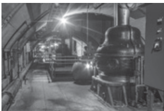
The Thrust Deck level of the station. The housings contain the thrust bearings that align the shaft between the dynamo and the turbine (Conlon 2019).
