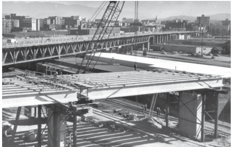
Fig. 6. Construction of new Georgia viaduct, with original viaduct in the background (Vancouver Express 1970)
