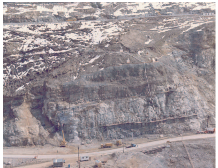
Fig. 1: Photo of the 731 Block shortly after remedial measures were completed in 1980. Photo courtesy of B.C. Hydro.
