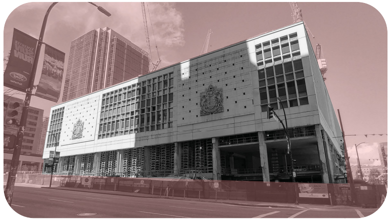
Vancouver Main Post Office - current condition under partial deconstruction - viewed from Georgia St. looking north-west
