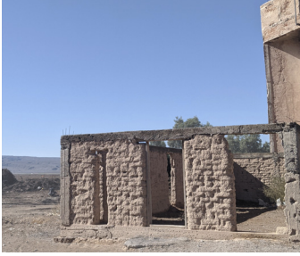
Traditional building method in concrete framing, infilled with adobe blocks and covered in cement parging.
