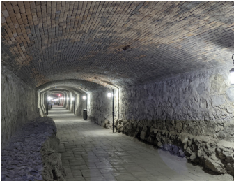
Stone masonry and cement parging widely used for canal lining and foundations.
