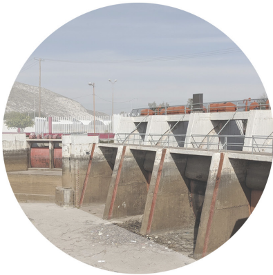
5 - San Fernando derivation dam Contemporary Systems
