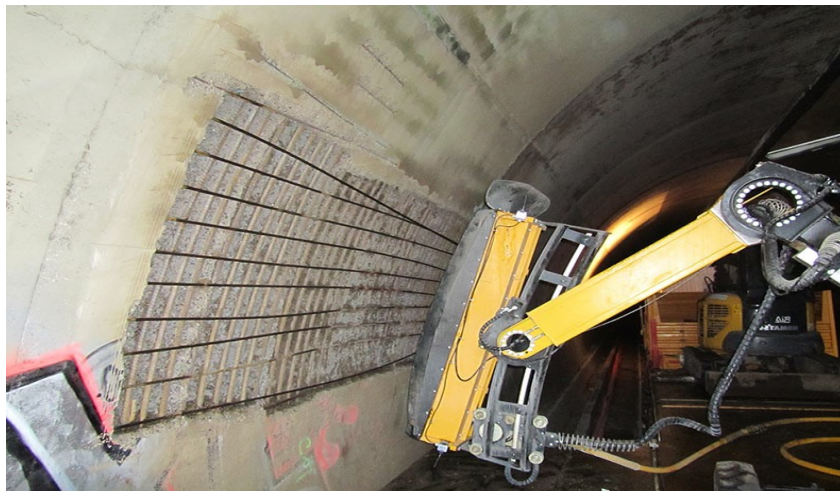
Figure 1- 1: An example of concrete deterioration in tunnels [10].
