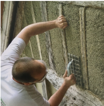
Figure 63: Hempcrete can be shaped with a nail or grid float after casting (Stanwix and Sparrow 2014, 188)
