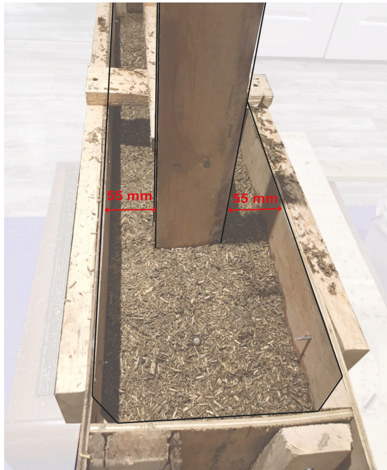
Figure 45: This structural frame is set in the middle of the wall to give maximum coverage of 55mm around the frame. This is above the recommended minimum for protection of the structural frame.
