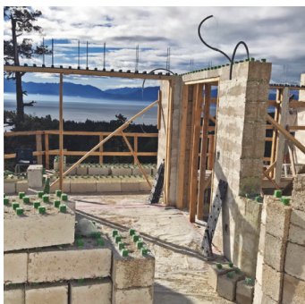
Figure 39: Hempcrete block home under construction using structural blocks. (JustBio Fibre Structural Solutions 2017)
