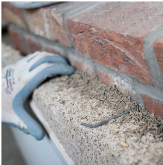
Figure 71: Hempcrete application against existing or new brick. This method is used for the demising wall between the extension engineering and the Hemp Research Centre. (ISOHemp 2020)
