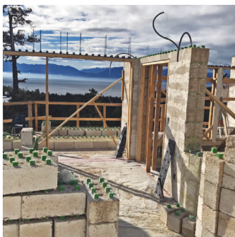
Figure 2: Hempcrete block home under construction using structural blocks. (JustBio Fibre Structural Solutions 2017)
