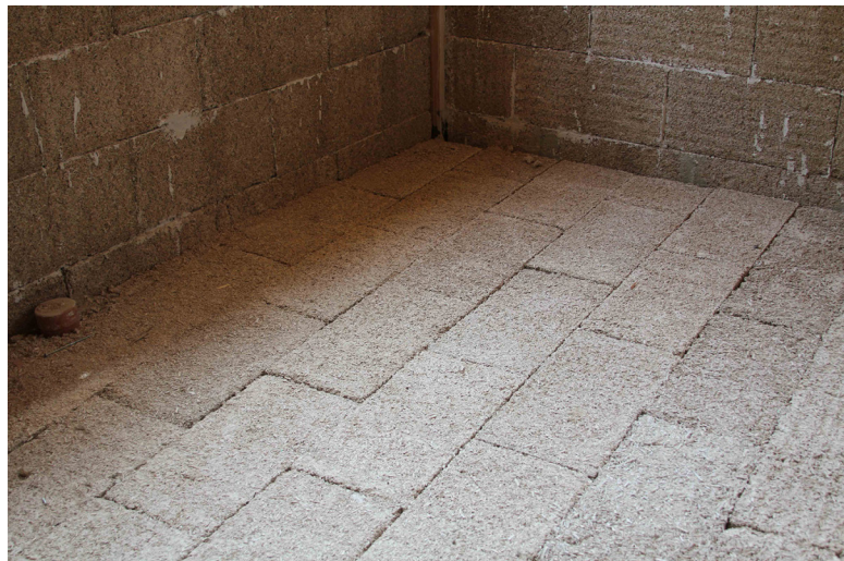
Figure 51: IsoHemp blocks used for insulation an subbase on the floor as well as the walls.
