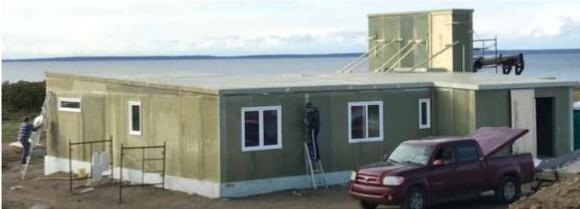
Figure 2-7 Meteghan River house under construction made using foam recycled from plastic (Comeau, 2019).
