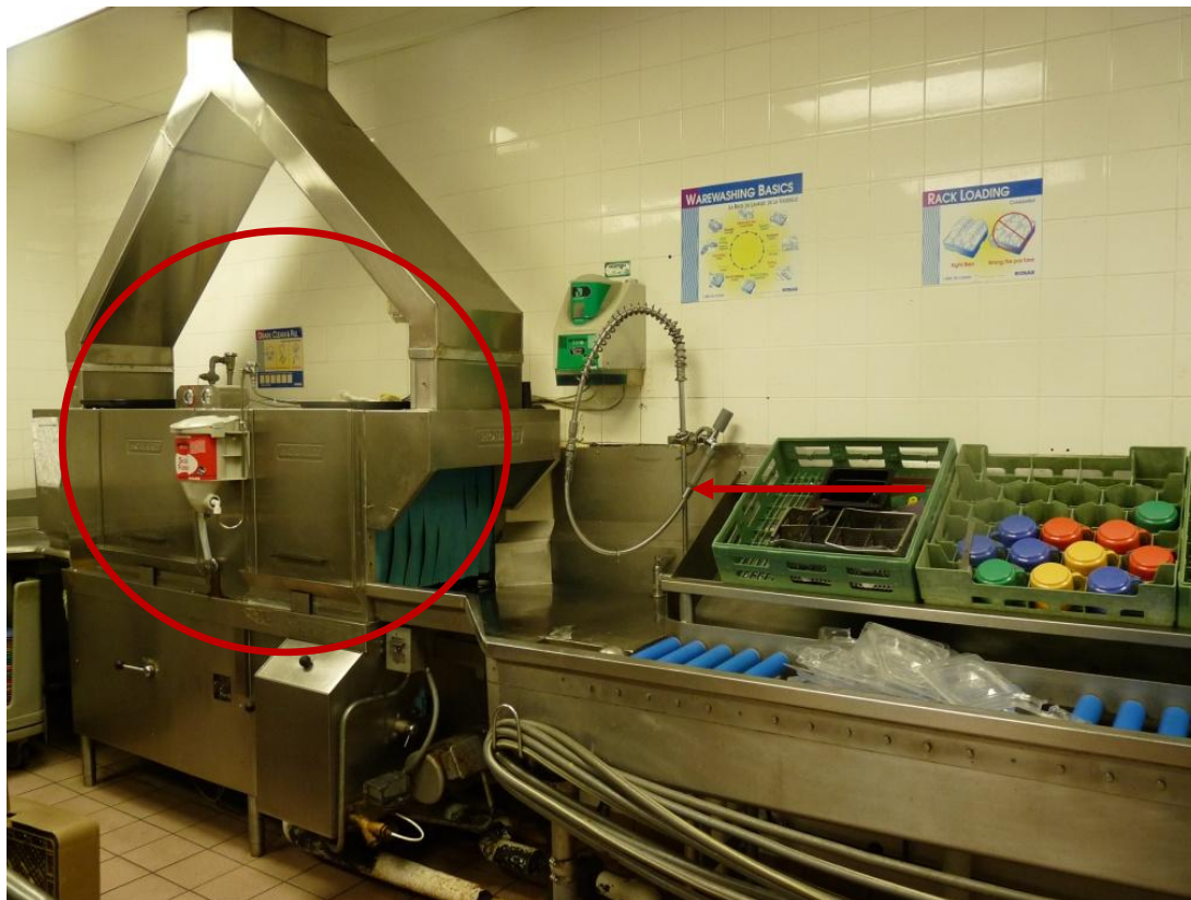
Figure 2: Riskey Hall's Dish-pit. The arrow points to the sprayer, the dishwasher is circled.
