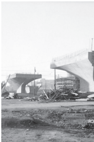
New Georgia Viaduct construction, 1970; photograph by Walter Frost, from the City of Vancouver Archives.
