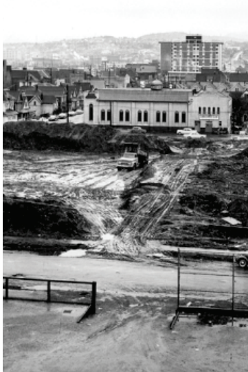
View of the Strathcona redevelopment work site for the Mau Dan Gardens, 1967; from the Maudan Co-op.
