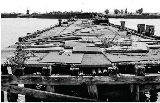
Abandoned and decaying industrial pier in the Erie Basin, Red Hook
