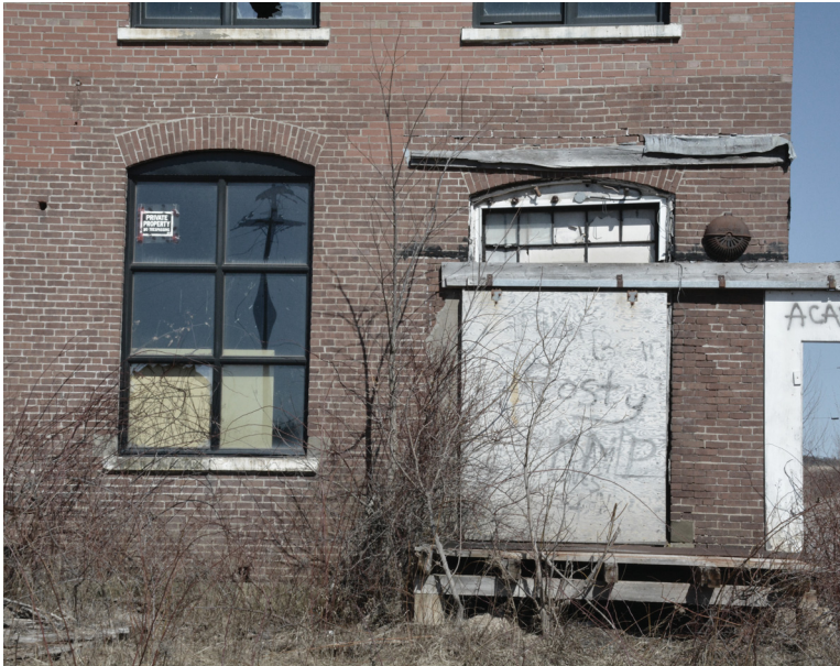
Photo taken on site of existing door condition. Platform above grade suggests flood plain foundation.
