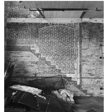
Photo taken inside existing mill. Observed trace of a previous stair before it was infilled and a building addition was added.
