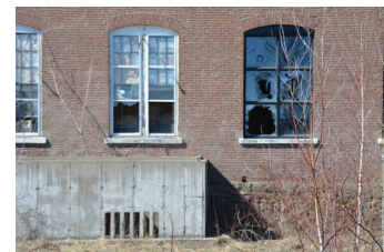
Windows as seen from the exterior. White frames are older than black frames as the black frames were installed during the failed redevelopment attempt in 2007. Photos taken March 2019.
