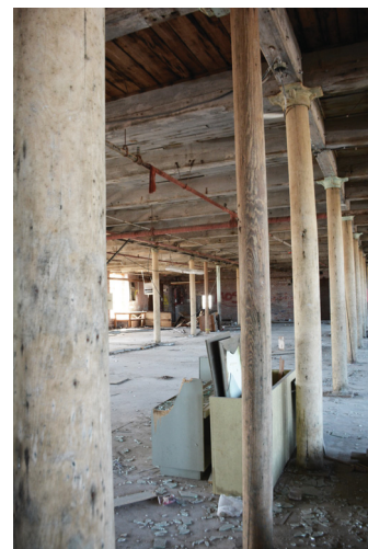
Wooden columns seen on ground floor of former Nova Scotia Textile Mill.
