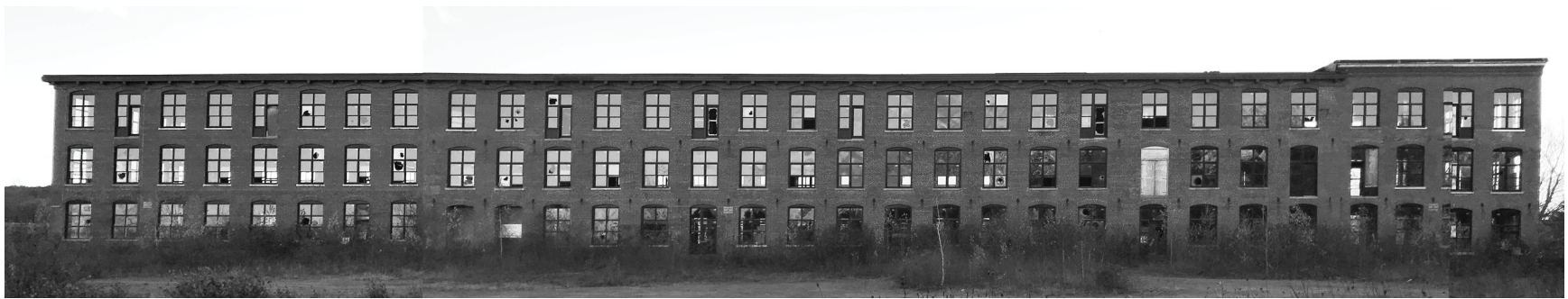
Stitched elevation of north facade from photos taken during site visit March 2019.
