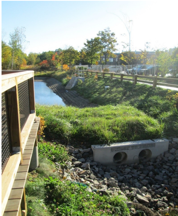
Figure 6.8.17: Pipes diverting stormwater from the forebay to the constructed wetlands. Saulnier, October 17, 2013.
