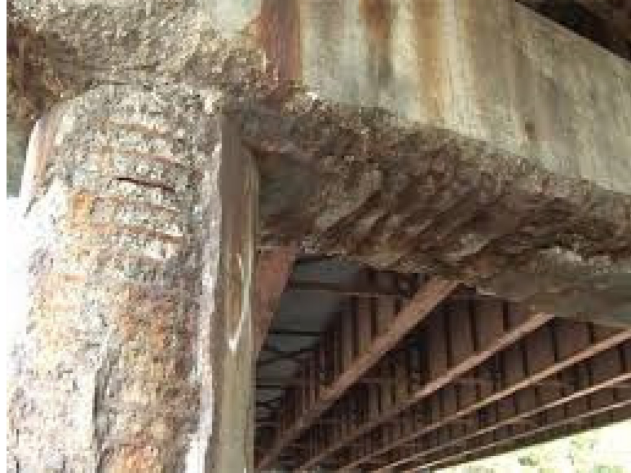
Figure 2.2 Corrosion deterioration of bridge structure
