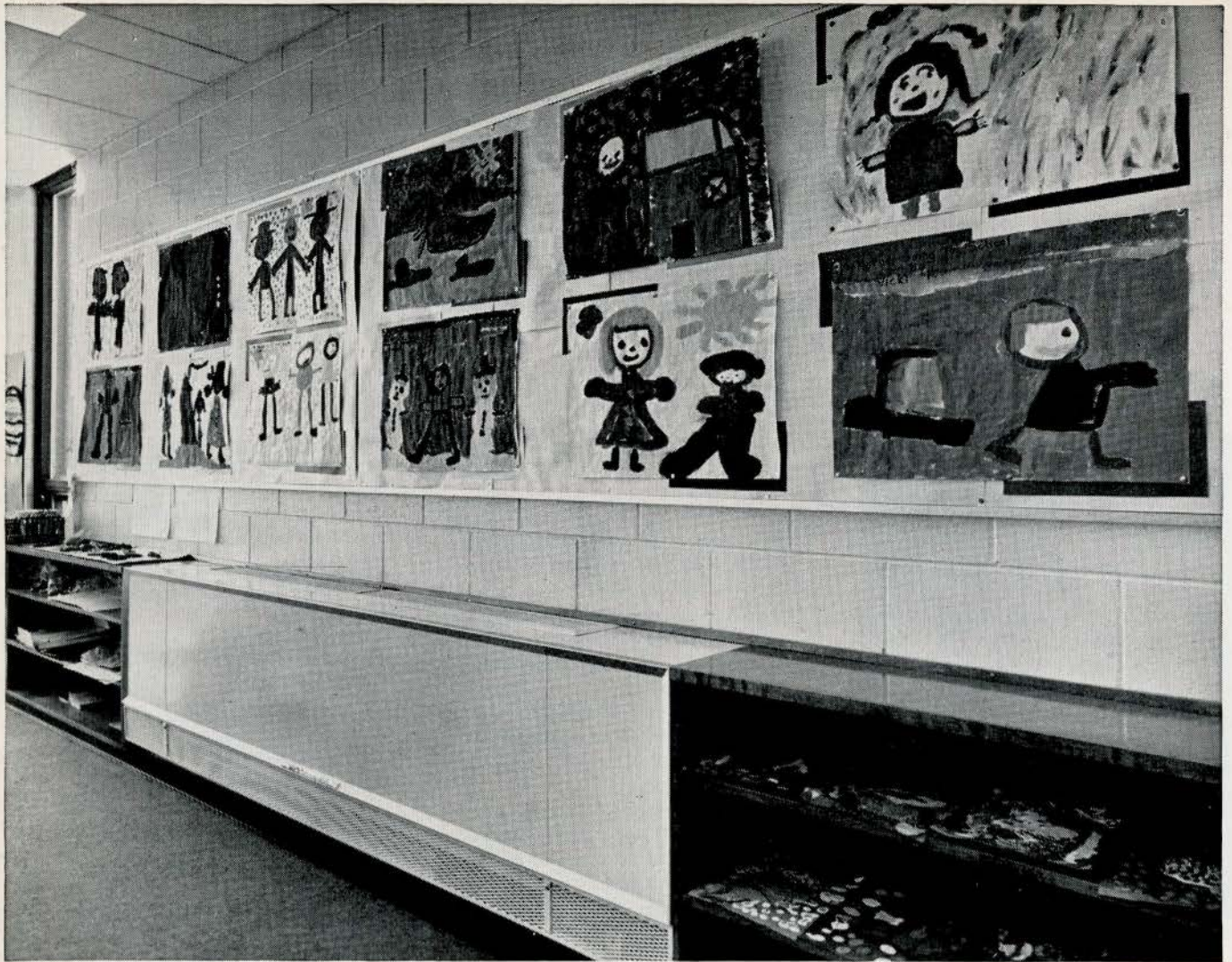
One of the electric unit ventilators at Redwood Public School. Architect: Jean-Paul St. Jacques, M.R.A.I.C. Consulting Engineer: Howard Boland, P.Eng.
