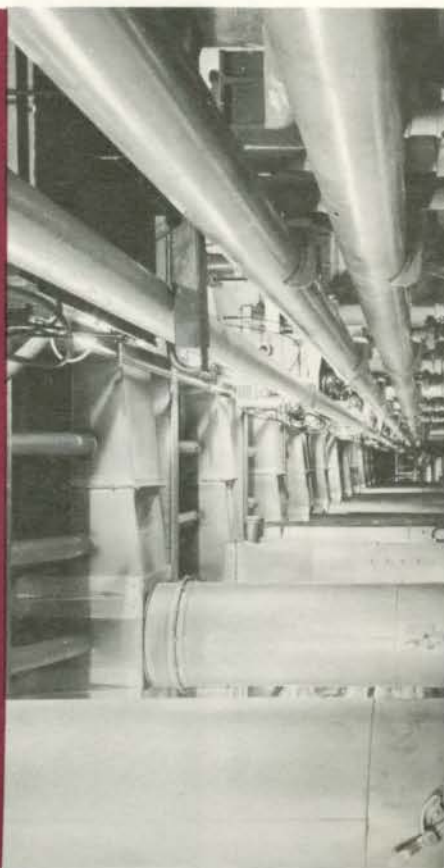
General view of the float bath/Pipework and ducts under the float bath
