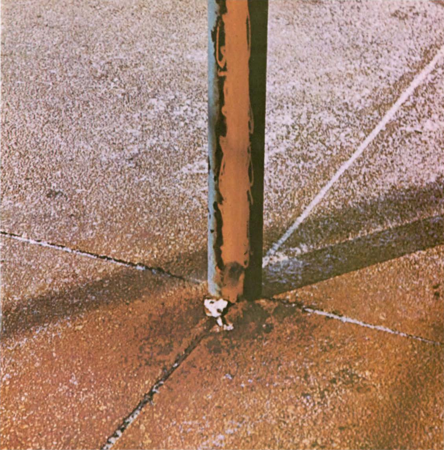
This pipe column supports the canopy of one of Montreal's newest and largest shopping centres
