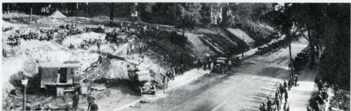
5. New Terminal Station was to have been an unemployment relief program. Shown is work progressing on Lagauchetière Street, east of the old Canadian Northern Station. CNR Photo
