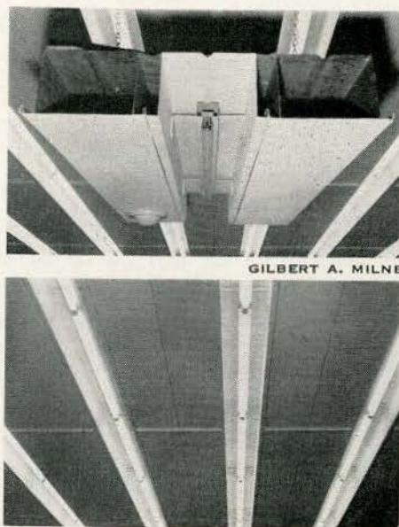
Top: section of steel roof deck construction showing air distribution ducts and lighting. Bottom, drafting room ceiling, Margison & Associates new building.
