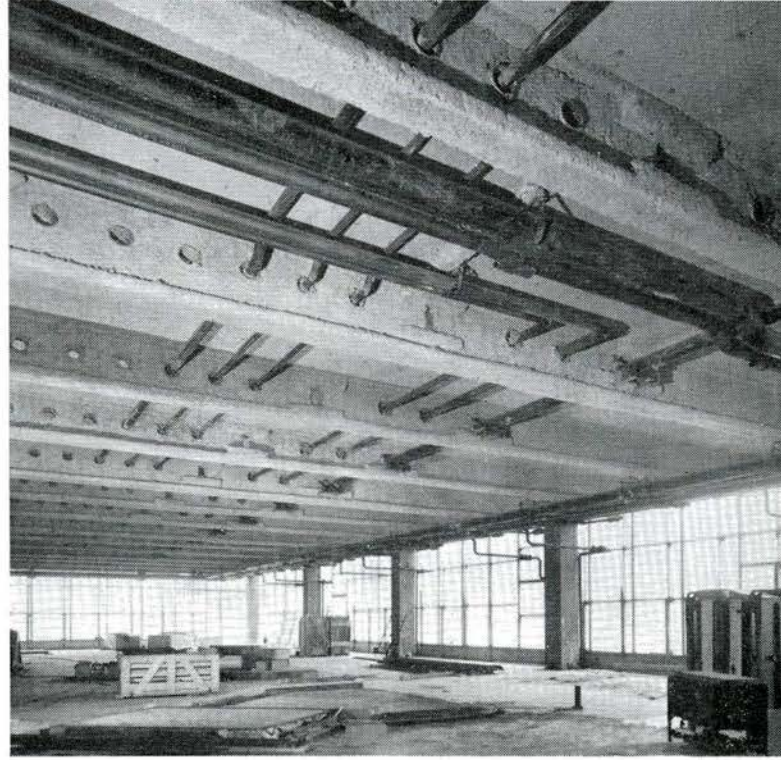
Steam and water pipes are carried through the steel.
