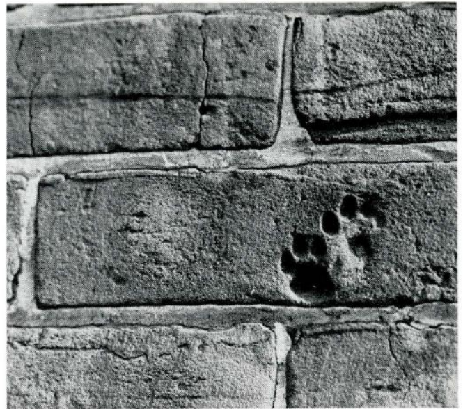
FIG 9 Cracks in bricks and mortar joints.
