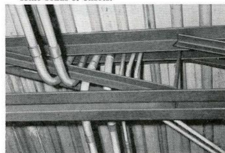
SMALL PIPES FOR OXYGEN, vacuum and electrical services are easily passed through the spaced double angle top chords of the joists directly into partitions without troublesome bends or offsets.
