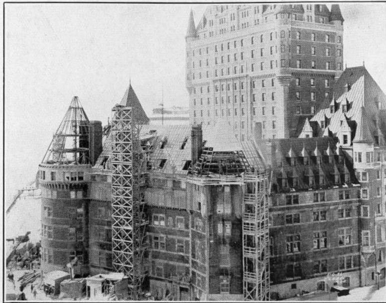
Here is a view of the Chateau Frontenac, Quebec, P.Q. where Precast Gypsum Short Span Roof Slabs were used in repairs following a serious fire.
