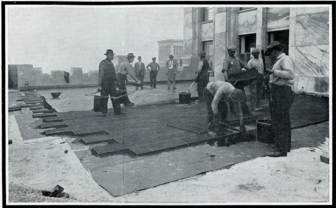
99,000 sq. ft. of Armstrong's Corkboard were laid on the roof of the Fisher Building, Detroit. Albert Kahn, Inc., Architect; J. D. Candler Company, Roofing Contractor.
