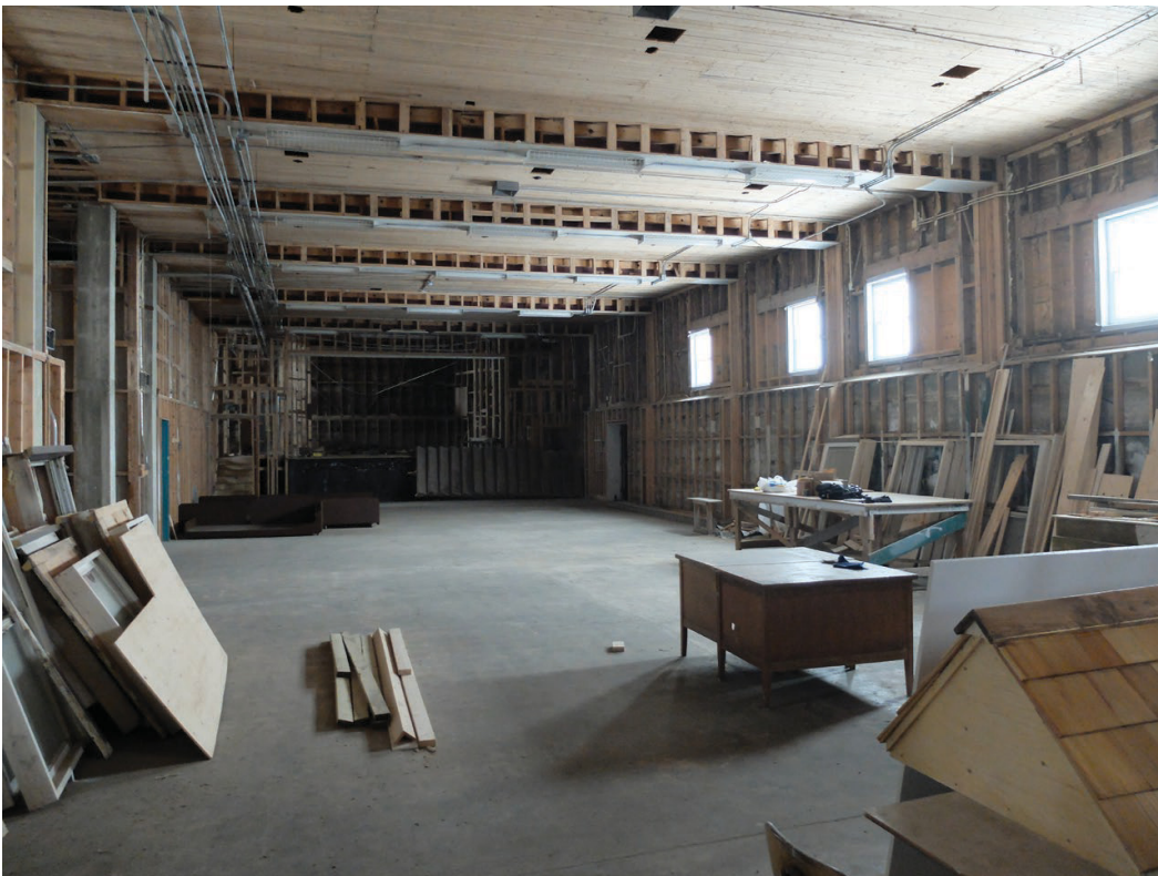
Fig.90 Interior photos of the existing building (second floor above, lower floor below).
