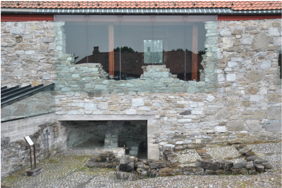
Fig.63 Exterior of the Hedmark Museum in Hamar, Norway, showing the clear distinction between old and new elements, carefully touching the partially restored existing building. The glass and wood components accentuate and highlight what remains rather than hiding or overwhelming it. Source: Umanskay, 2014.
