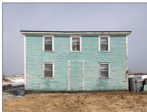
BUILDING WITH PAINT DETERIORATION, RUST FROM NAILS, AND EVIDENCE OF A FAUX FRONT DOOR
