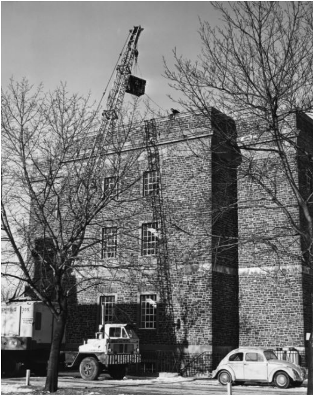
Hoisting the new IBM 1620 into place at the top of the Dunn Building, March 1964.
