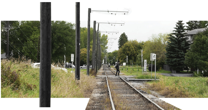
As found neglected conditions along railway line.
