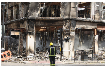
Destruction of union point building (Spectator 2011)
