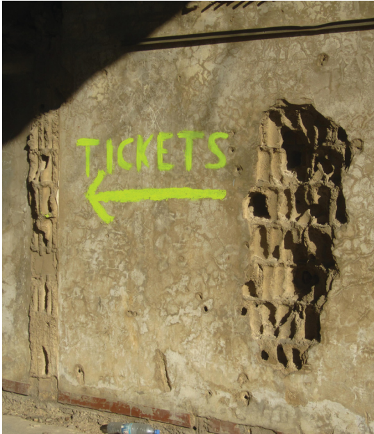
Damaged and graffitied wall, Beirut, 2015
