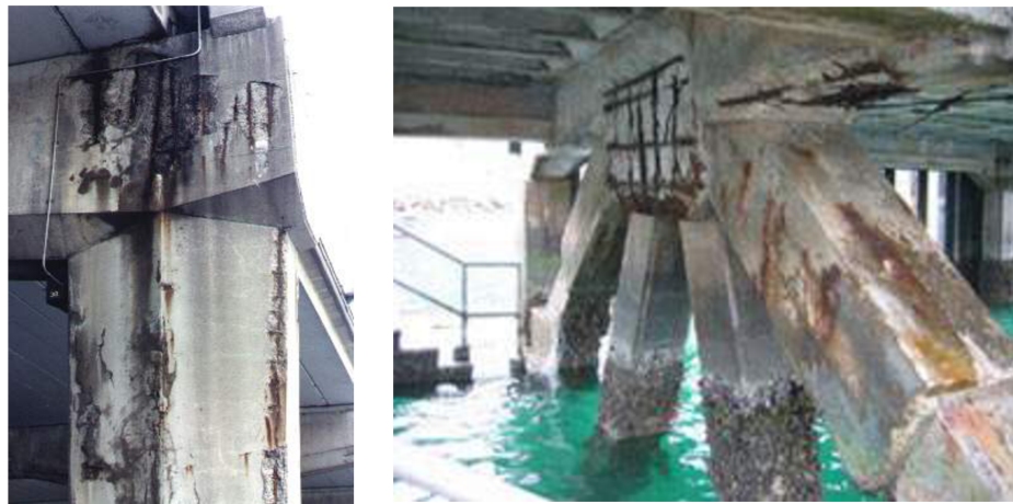
Figure 2.6 Heavy delamination and corrosion damage in reinforced concrete structures exposed to marine environments [21]
