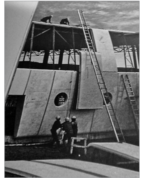
FIG. 12. ASSEMBLING OF PREFABRICATED PANELS FOR THE GORDON ROBERTSON EDUCATION CENTRE. | REPRODUCED FROM PGL ARCHITECT, ARCHITECTURE DE PGL 1959-1975 , MONTREAL, 1975 (N.P.).
