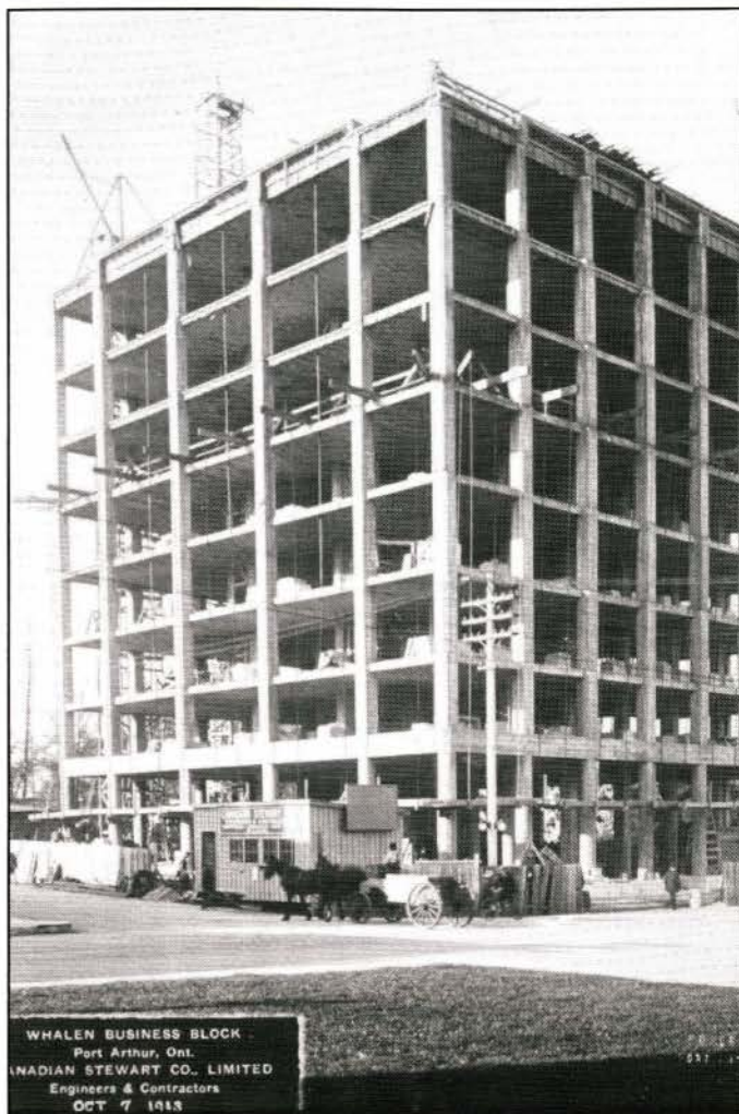
Figure 2. Construction photograph of the Whalen-Hydro Building, 7 October 1913. (Whalen Archives, Norman M. Paterson Library, Lakehead University)
