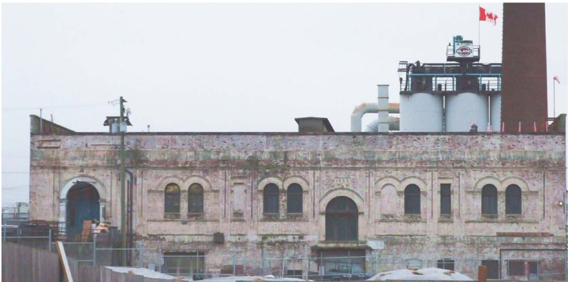
Picture of the 1892 Powerhouse Building (Wilson 2015), which is restored and converted into a community centre.
