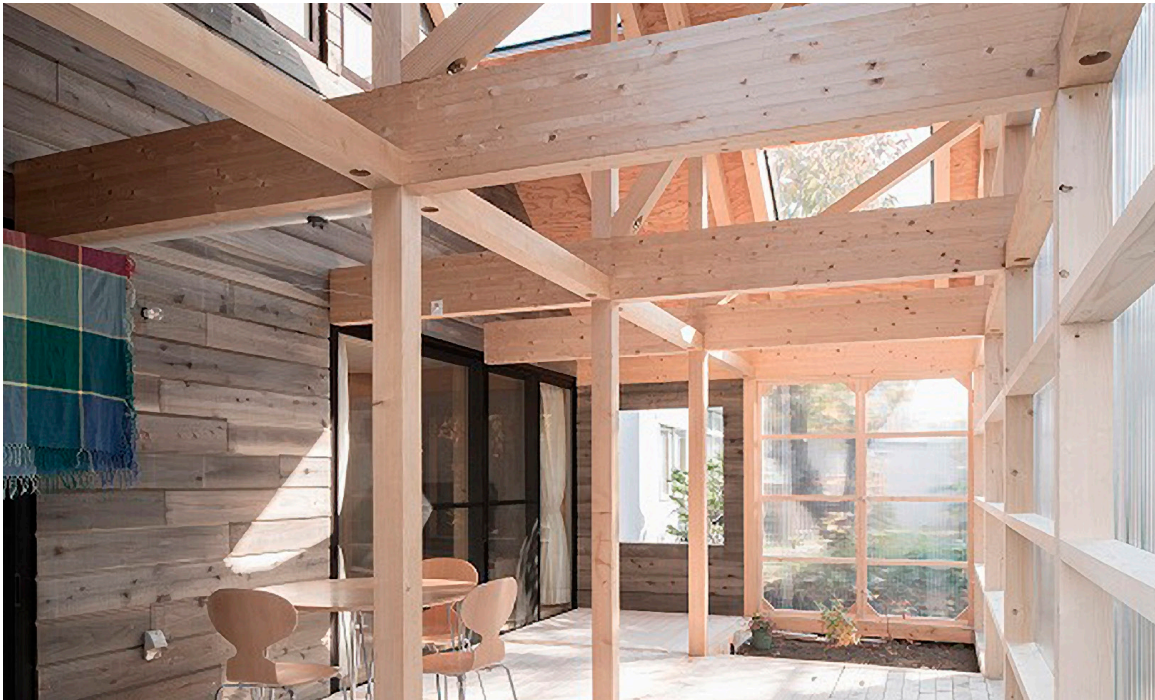
Figure 44. Enclosed winter garden; showing a combination of shear walls and moment frames as a mixed system, 2011; from Yoshichika Takagi + Associates.
