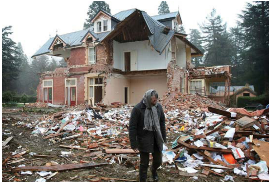
Figure 14. Collapsed masonry house devastated from seismic forces, 2011; from Christchurch City Libraries.
