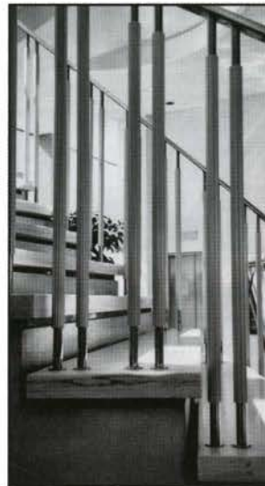
Fig. 33. Detail of the stairwell's stainless steel balustrade, and marble steps and risers. (A. Waldron, HSB, 2001)
