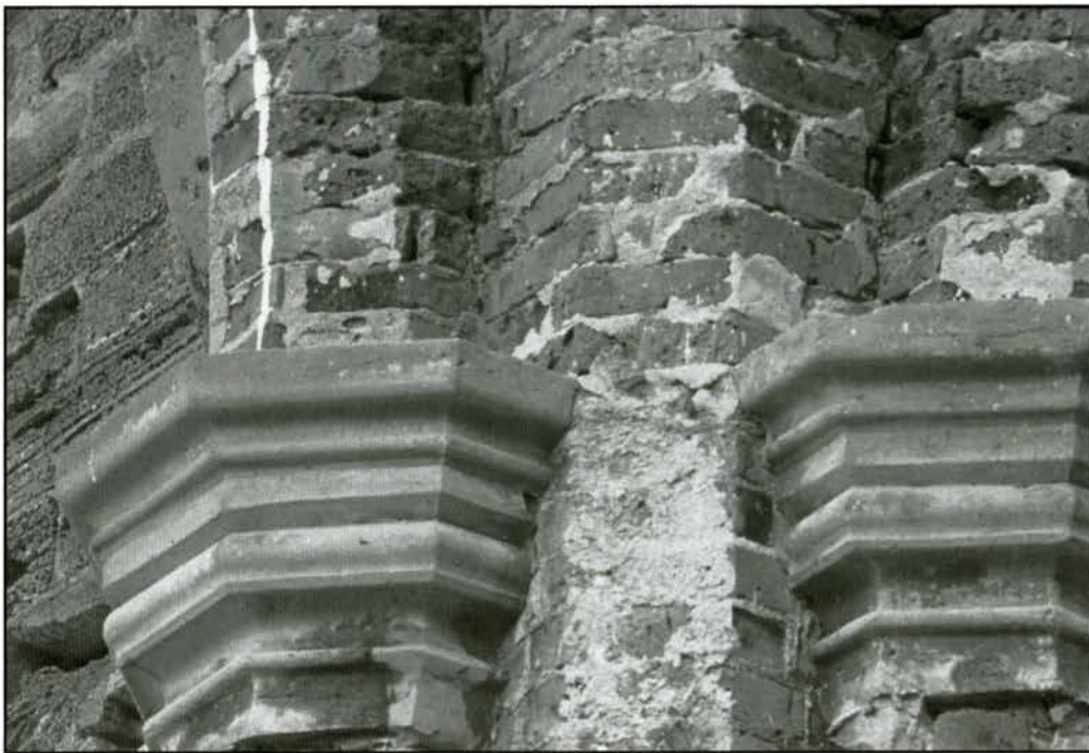
Fig. 10. St. Peter's, "The Unfinished Church", St. George's, Bermuda. Tower pier composed of red brick. (Photo: Barry Magrill)
