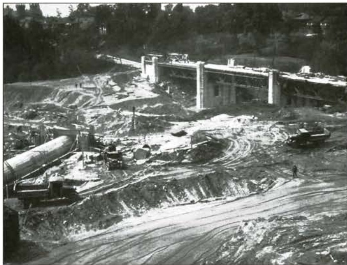
FIG. 7. VIEW OF RESERVOIR AND BRIDGE UNDER CONSTRUCTION. | PHOTO: ARTHUR GOSS, CITY OF TORONTO ARCHIVES, RGB, SERIES 65, ITEM 71
