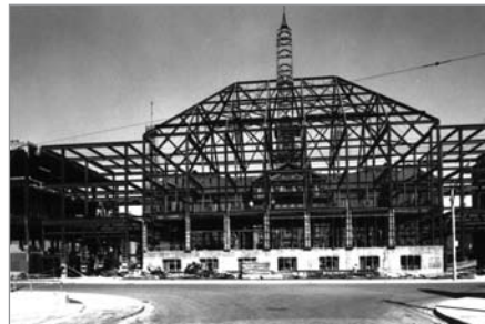
FIG. 12. KERR HALL UNDER CONSTRUCTION TERMINATING THE NORTH END OF BOND STREET. | RYERSON UNIVERSITY ADVANCEMENT.
