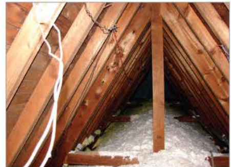
FIG. 27. ST. PAUL'S ANGLICAN CHURCH, KINGSTON, ROOF AND SUPPORT BEAMS TOWARD THE EAST. | PAUL CHRISTIANSON, 2010.
