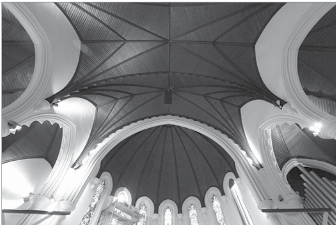
FIG. 27. NEW ST. PAUL'S ANGLICAN CHURCH, DETAIL OF THE CUSPED TRANSVERSE ARCHES AT THE EAST END. | LORYSSA QUATTROCIOCCI, NOVEMBER 21, 2014.
